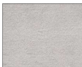
FB02 BETON MALOJA
